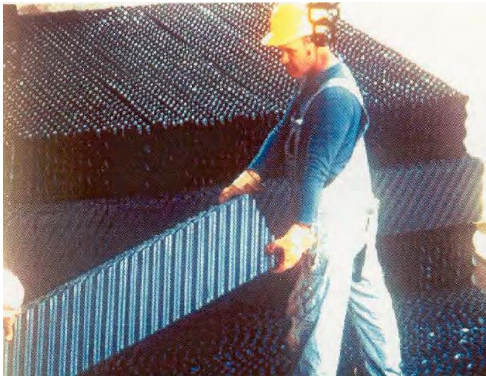
Figure 11 High-efficiency cooling tower film fill
